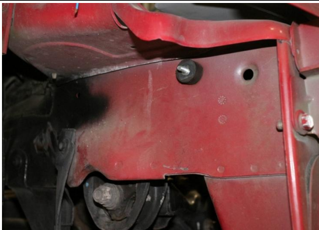
16. Install the 1/2" rubber mount onto the threaded hole on the frame rail behind the passenger side headlight.
